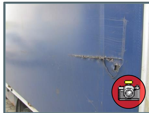
Tearing of siding
